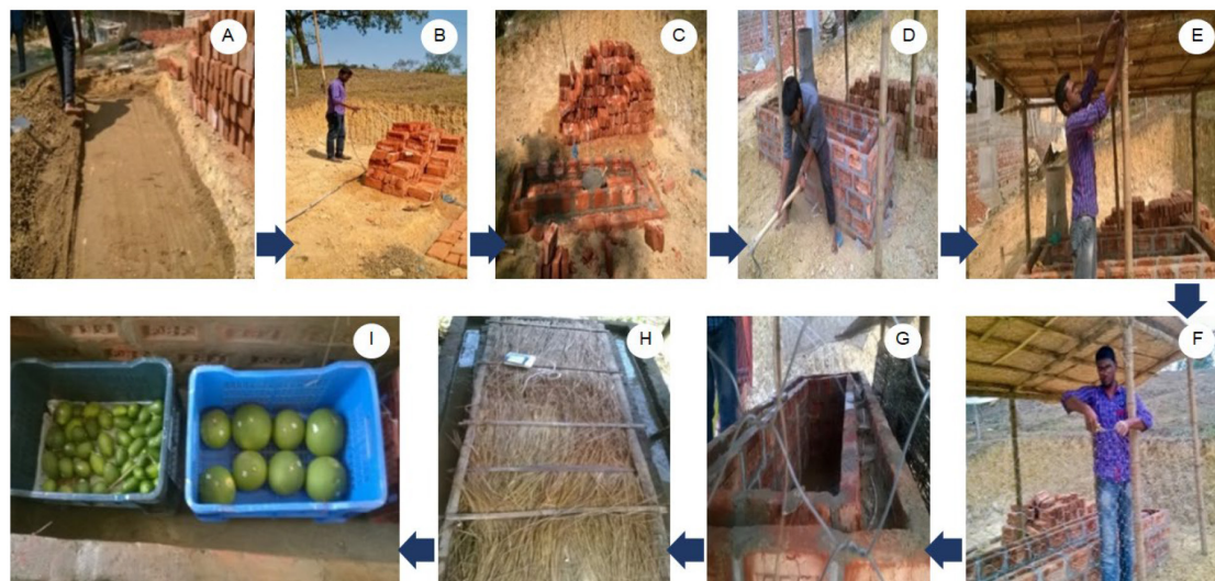
Figure 4 Construction of evaporative cooling storage structure (ECSS): (A) levelling of the floor space, (B) watering of bricks, (C) building of ECSS, (D) levelling of the soil around the structure, (E) shading for the whole structure, (F) fencing around the structure, (G) complete ECSS, (H) covering for the ECSS, (I) sample fruits in a crate
