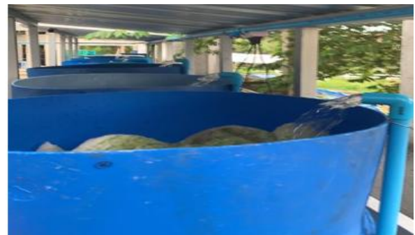
1c. The waste filtration system consists of fiberglass filter cloth and oyster shells and is installed in each fish tank.
