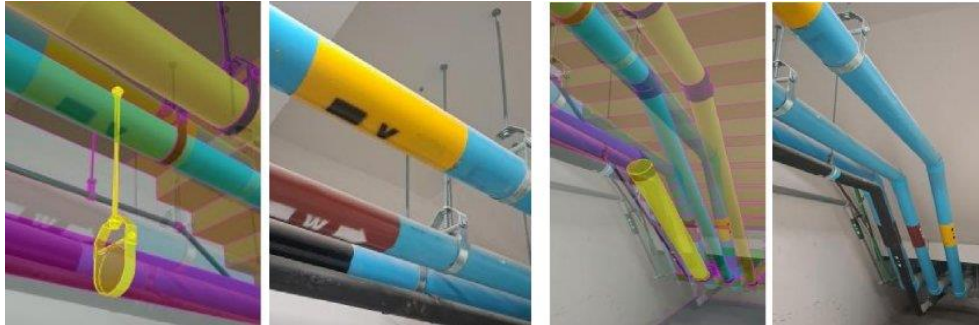
Figure 5 AR overlay of the sanitary piping system showing alignment issues between the BIM model and actual installation, particularly in pipe slope, hanger positions, and support fixtures.
