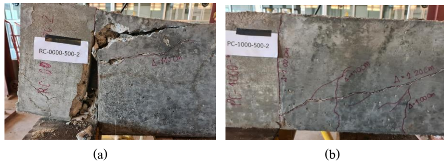
Figure 11 Failure of the beam specimen Group 3:
