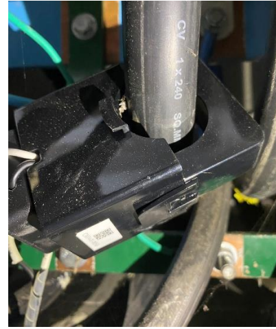
Figure 1 Clamp-on current measuring device (Clamp Meter) installed on a feeder conductor inside the Main Distribution Board (MDB).
