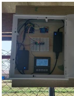
Figure 2. Box for control equipment and reporting parameters to smartphone
