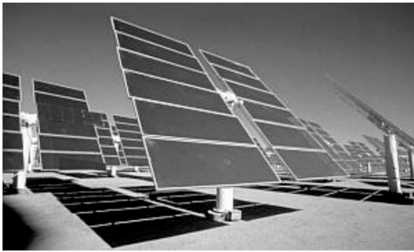
Figure 4 PV tracking system
