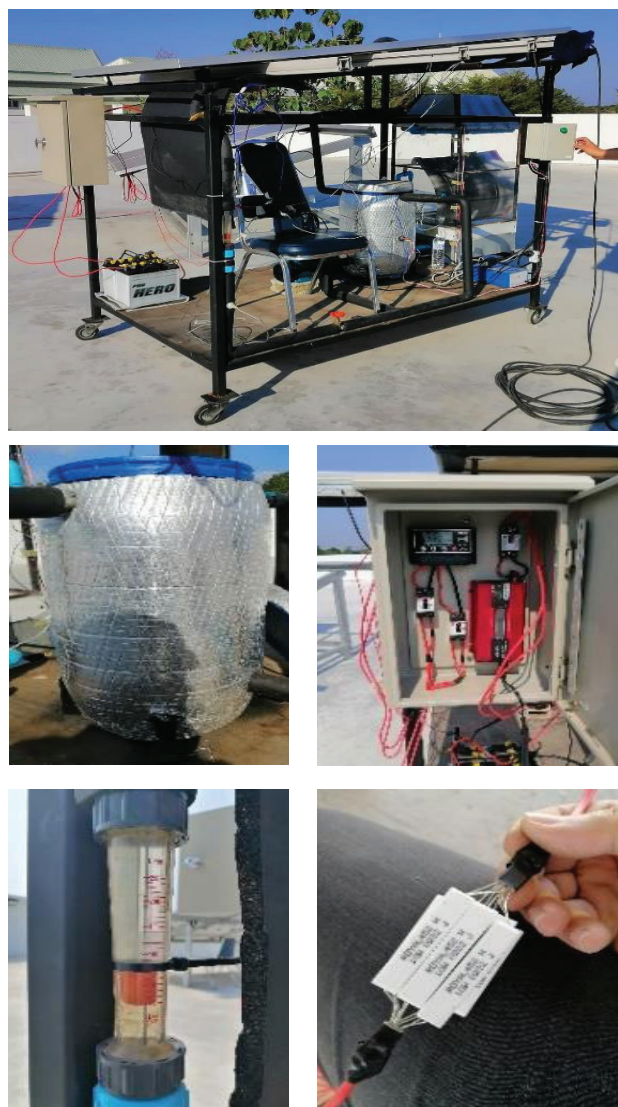
Figure 7 Examples of installed tools
