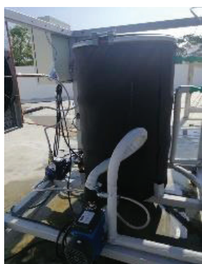
(c) Storage tank
