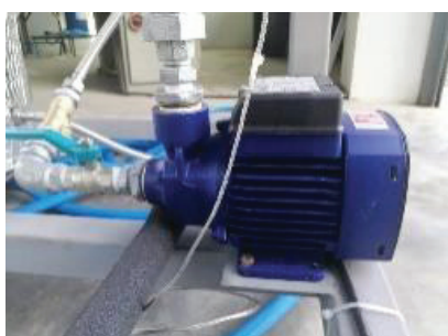
(e) Water pump
