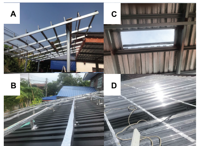
Figure 3 A solar collector structure.
