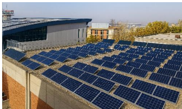
Fig. 14 Rooftop solar panel installation on the Ayaslı smart building at METU, demonstrating the integration of renewable energy technologies in sustainable campus infrastructure
