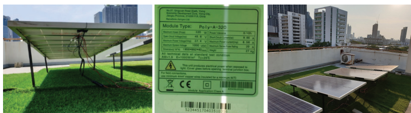
Figure 4 Solar panels for performance testing
